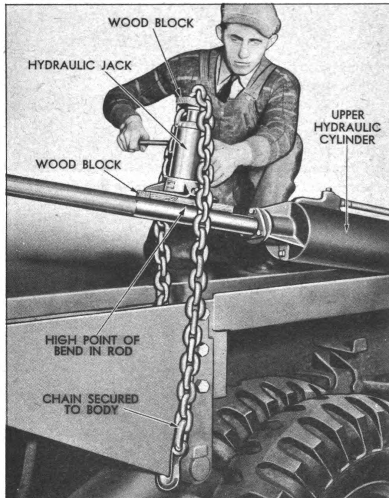
Figure 37. Straightening Rod from Above. Note Position of Wood Block to Prevent Marring the Rod. Method of Securing Chain to Body is Also Shown.
