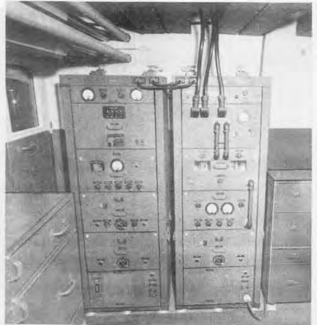
Range Transmitters installed in forward part of truck.
