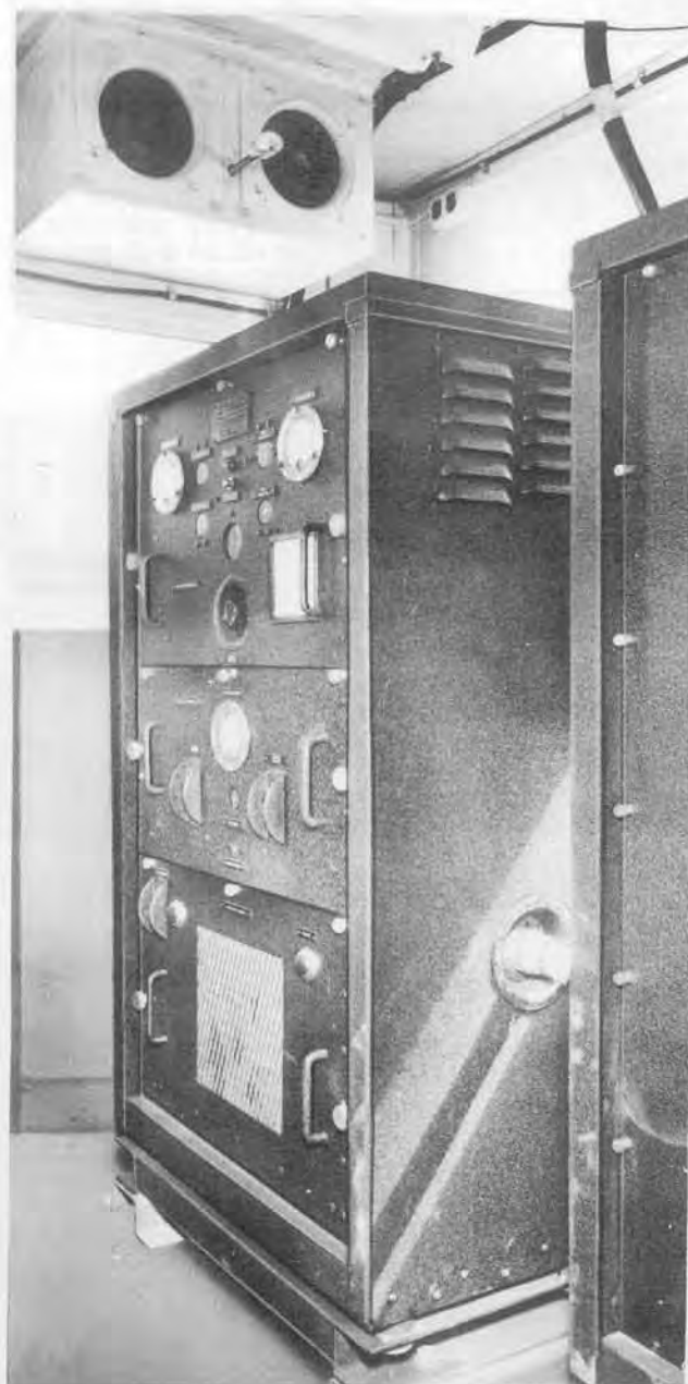
Radio Transmitter BC-751 installed in truck.
