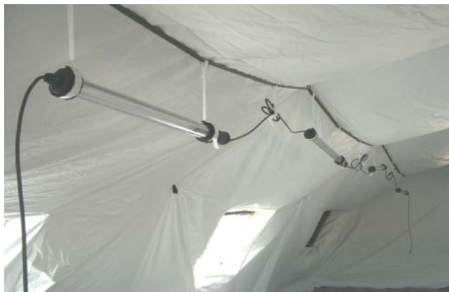
Figure 30. Lighting Unit Installed.
