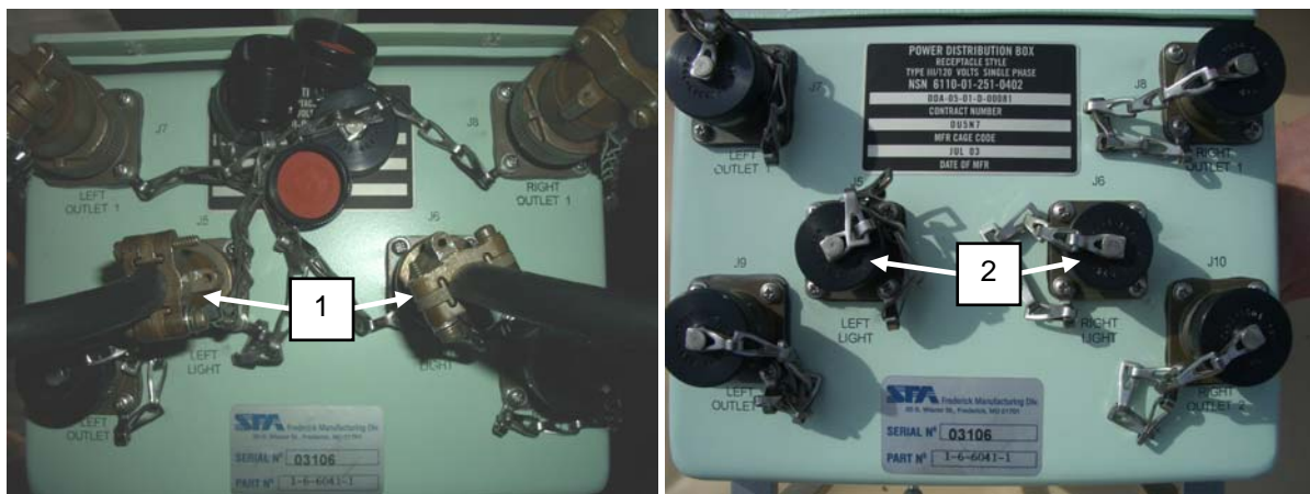
Figure 5. Disconnect Lighting Cable Plugs.
