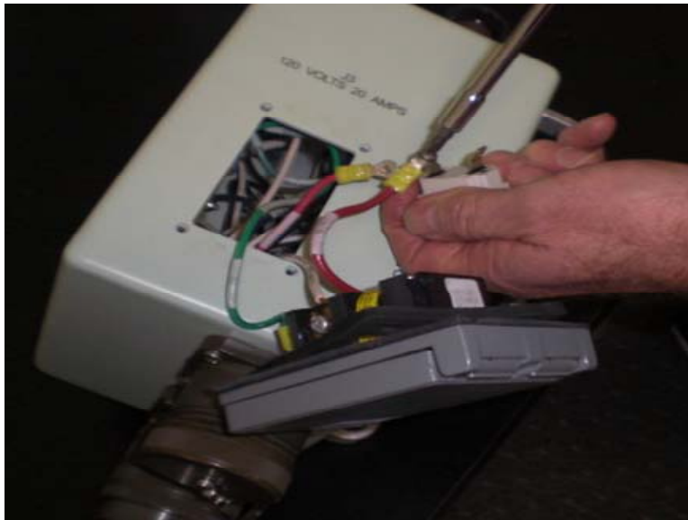
Figure 14. Disconnecting Circuit Breaker Wiring.
