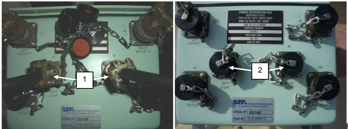
Figure 2. Disconnect Lighting Extension Cord Plug.
