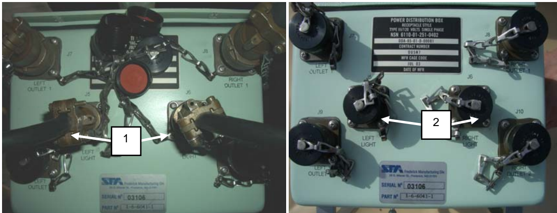
Figure 7. Disconnect Lighting Cable Plugs.
