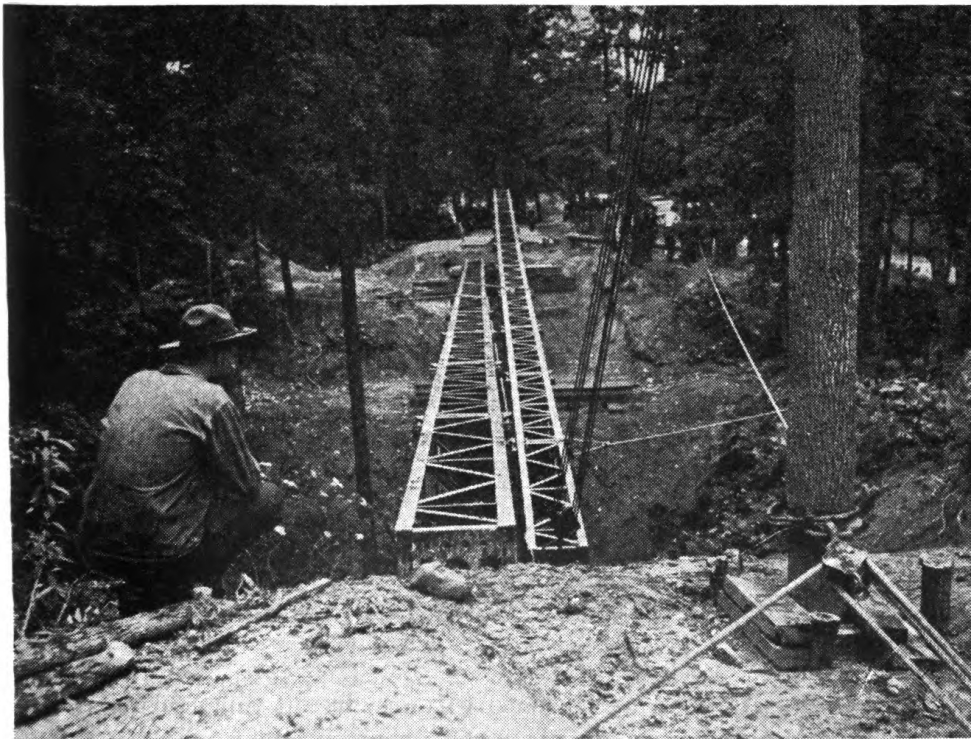
FIGURE 74.—Placing second girder. (Note gin pole in foreground, guide lines on girder, wire rope leading across ravine to tractor in background, and crane used for unloading sections.)
