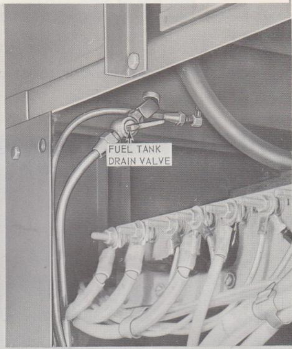
D. FUEL TANK DRAIN VALVE.
