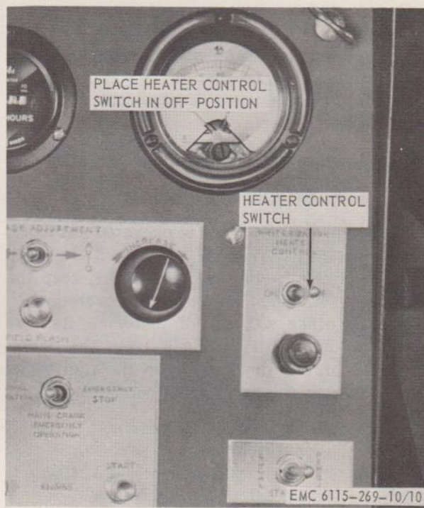
Figure 10. Winterization heater, stopping.
