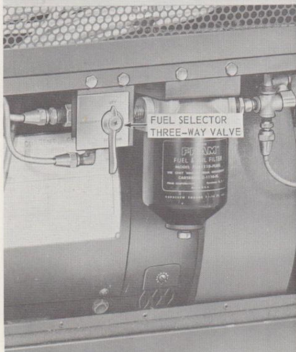
E. FUEL SELECTOR THREE-WAY VALVE
