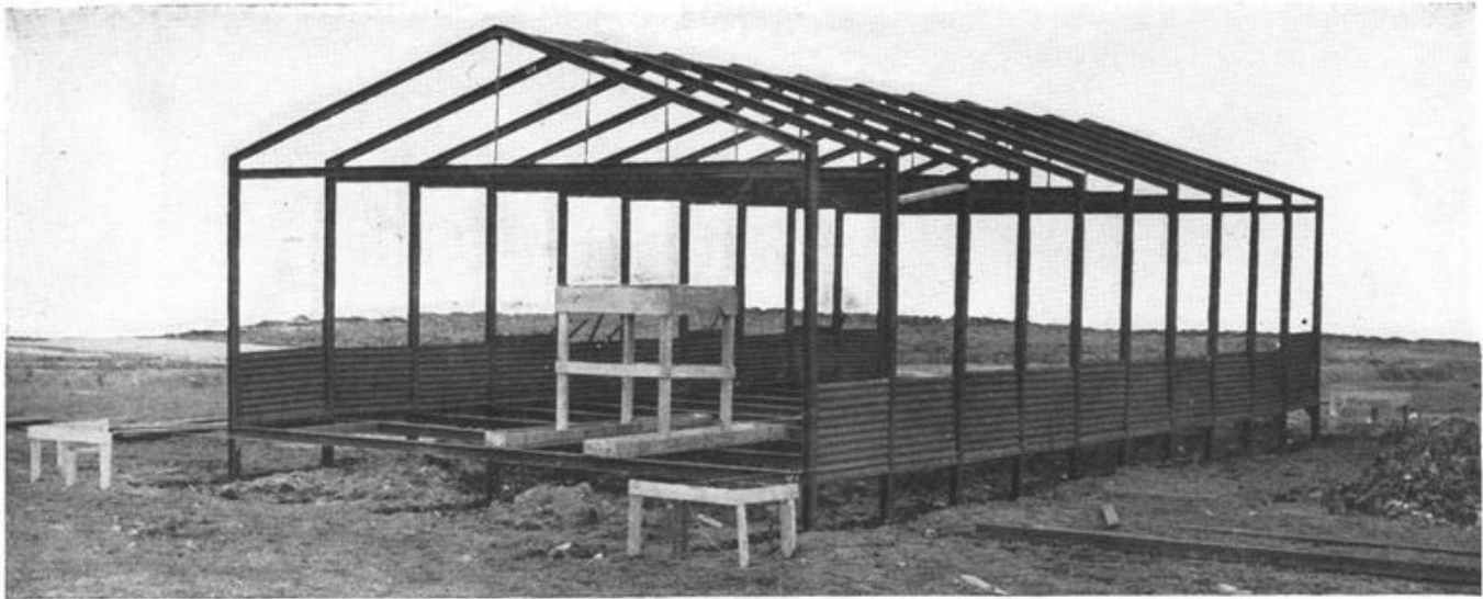
Figure 21. View showing wall panels grouped and placed into position. Note method of spreading ribs at eave to insert panels.
