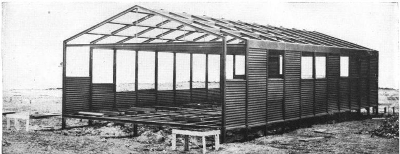
Figure 22. Eave angles with floor and roof purlins in place and some wall panels raised into position.
