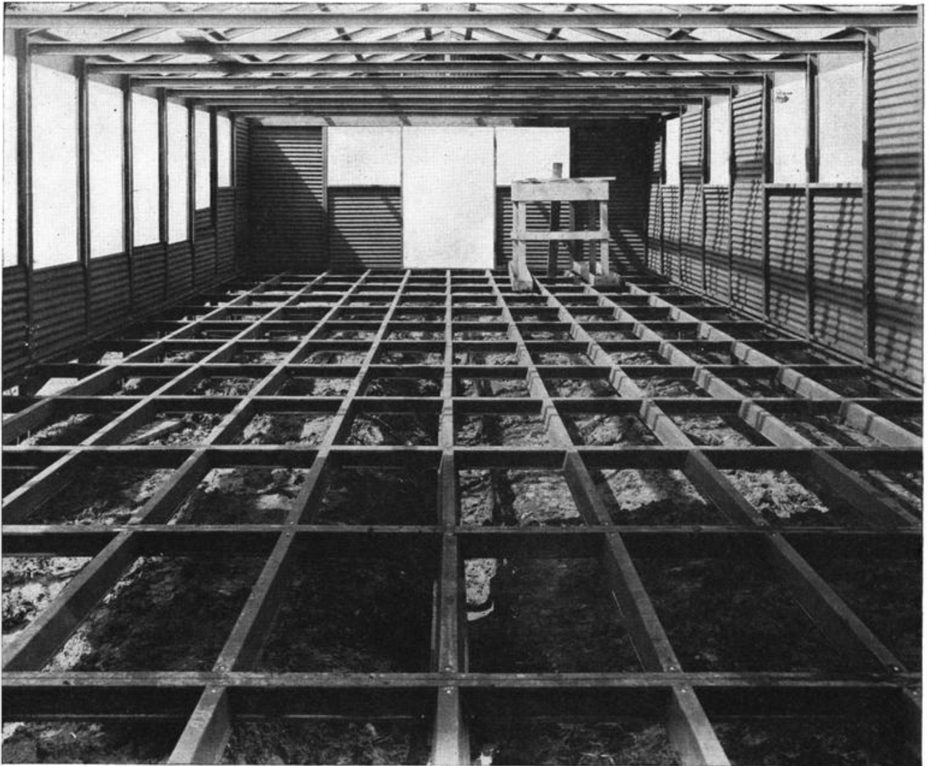
Figure 23. Roof and floor purlins in place. Interior view of erected building ends.
