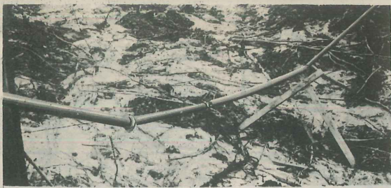
FIGURE 3 - This portable pipe line may look like a rail fence, but it gets the gas to where it's needed.
