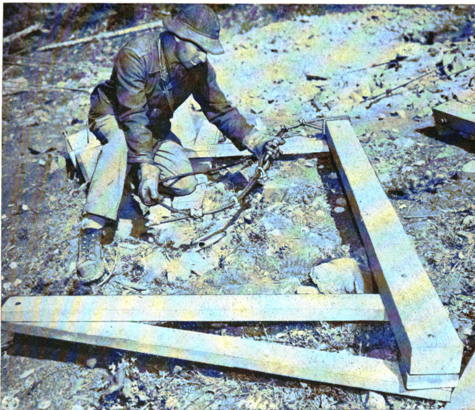
FIGURE 26. Assembled hanger. Hanger is assembled on near side and given to far side party to be installed.
