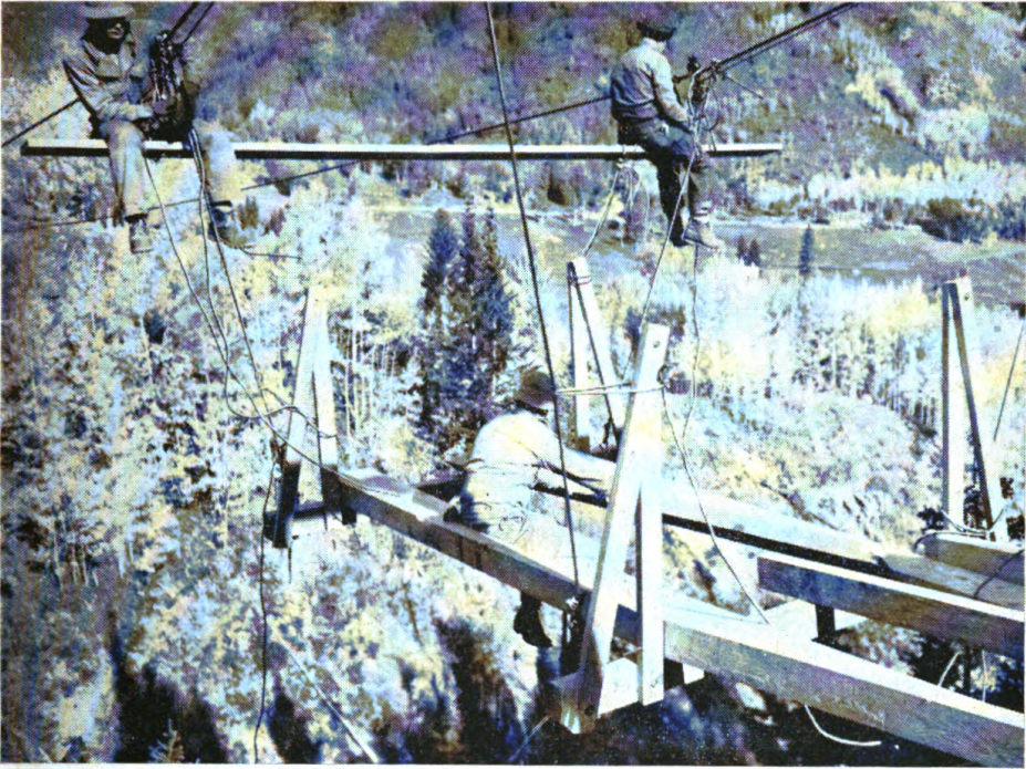
FIGURE 30. Placing stringers. Stringers must be placed from temporary scaffold plank. After the stringers are placed and nailed into position, the erection-scaffold party receives next hanger assembly and goes forward to next panel point.
