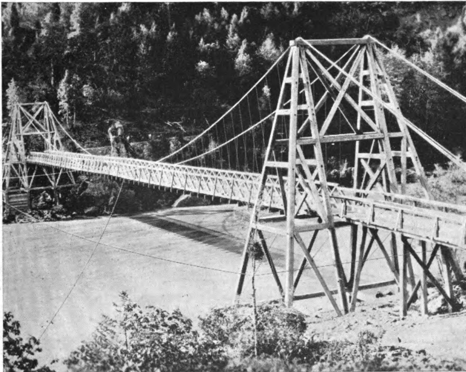
FIGURE 51. Pack-train suspension bridge. Used when a heavy type of bridge is required for mule traffic. Note tower design.
