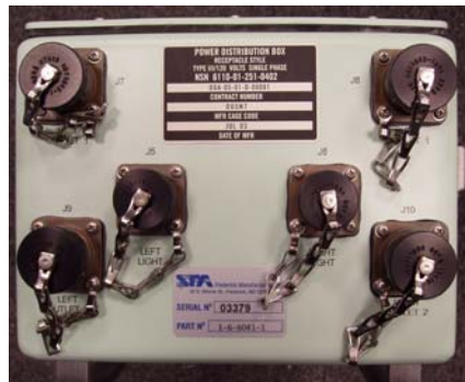
Figure 2. Power Distribution Box, Bottom.
