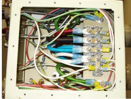
Figure 2. Distribution Box - Back Plate Removed.
