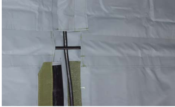
Figure 59. Cable Management System in the Ceiling in the Open Position.
