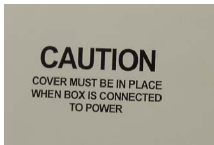
Figure 64. Caution on Power Distribution Box Cover.
