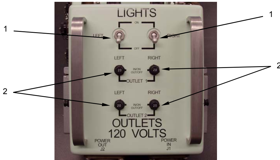
Figure 1. Switches and Breakers.
