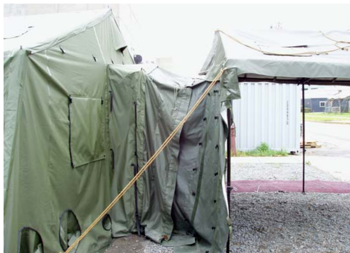
Figure 15. Connecting the Sandwich Wall to a Rigid Wall Shelter (RWS) Boot Wall.
