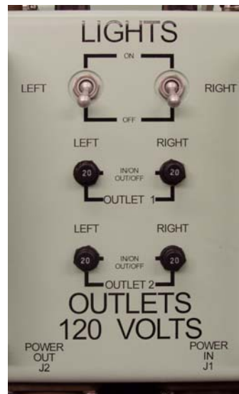
Figure 65. Decals on the Face of the Power Distribution Box.
