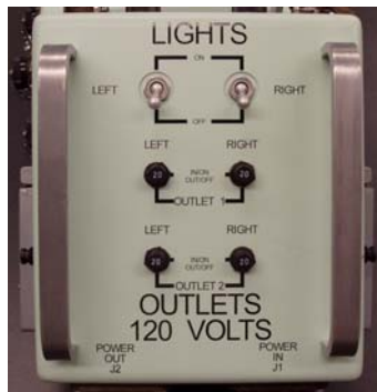
Figure 1. Power Distribution Box, Face.
