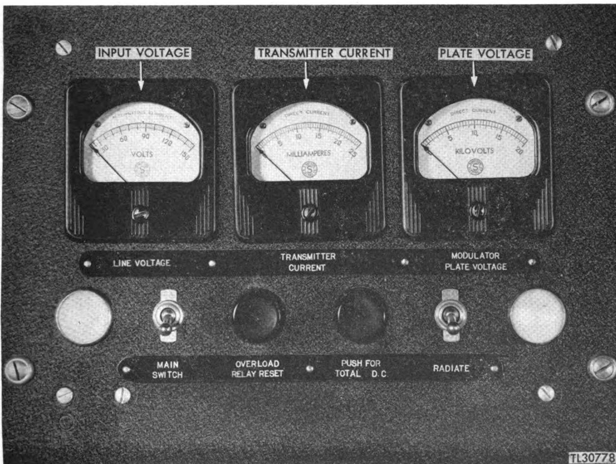
Figure 60. Transmitter cabinet control panel.
