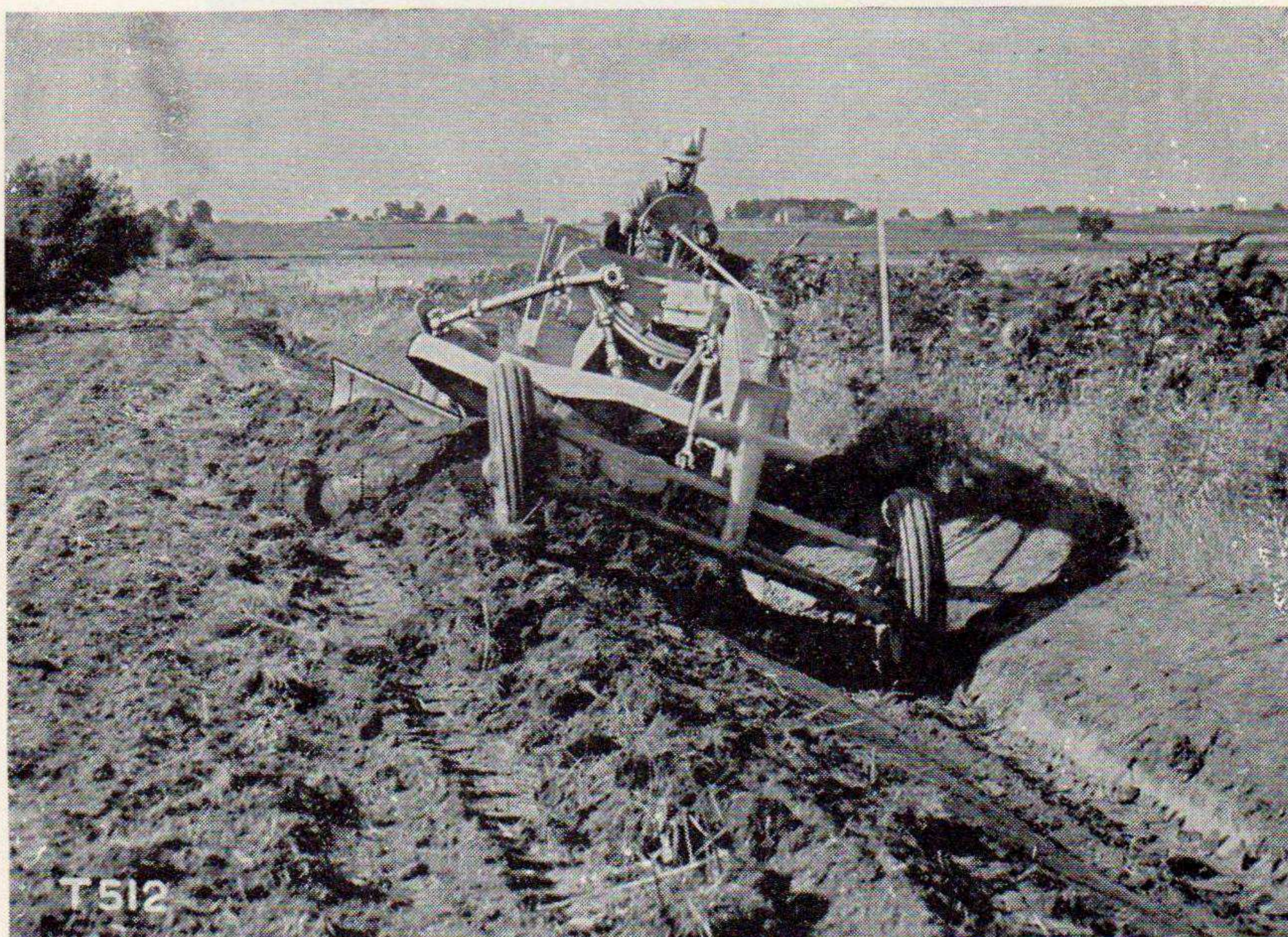
Figure 40. Cutting a trench on the inside slope is the first step in making a flat bottom ditch.
