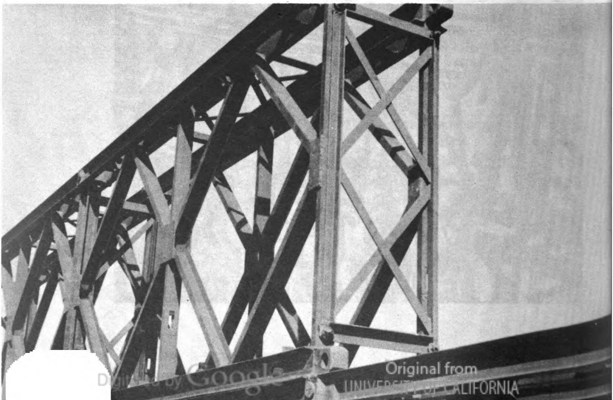
Figure 65.—Bracing frame placed vertically on ends of intermediate pair of panels on double-story bridge.
