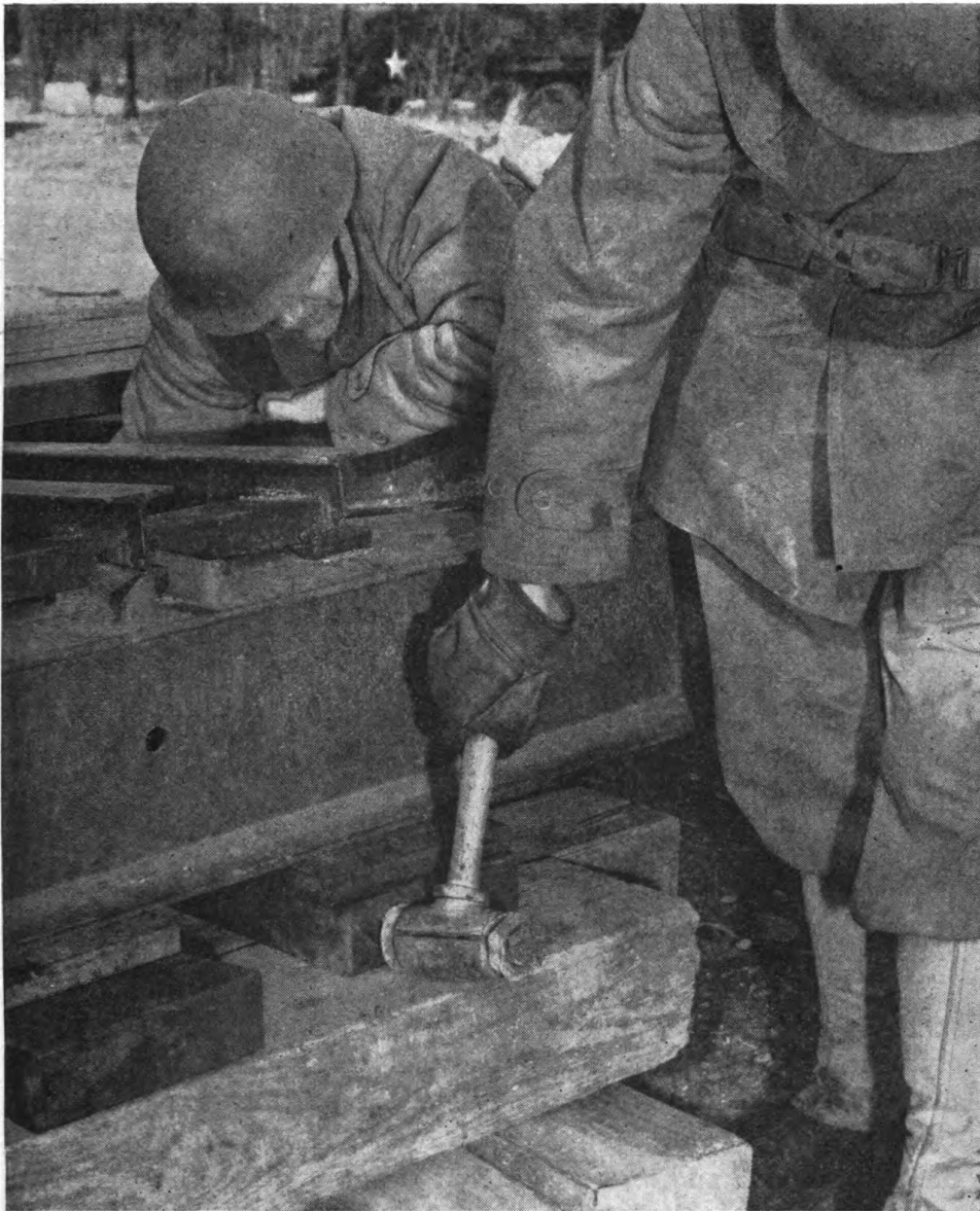
Figure 57.1.—Cribbing and wedging end transom at midpoint to carry loads exceeding 28 tons.
