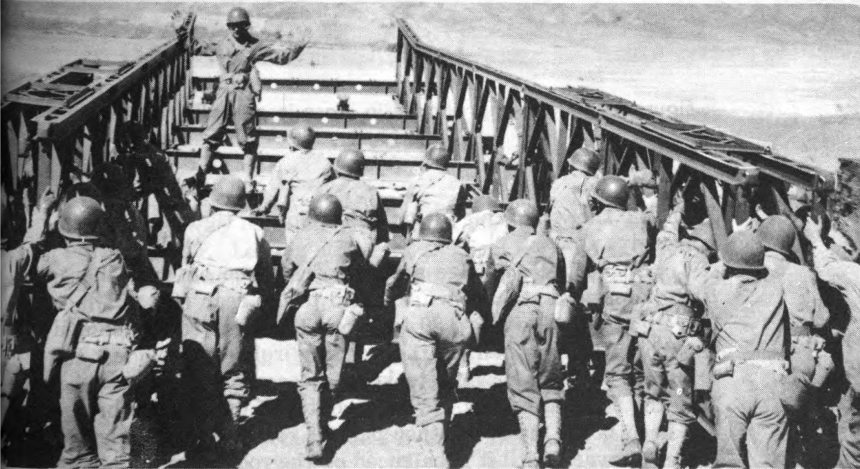
Figure 49.—Pushing launching nose over gap after completion of first two bays of bridge.
