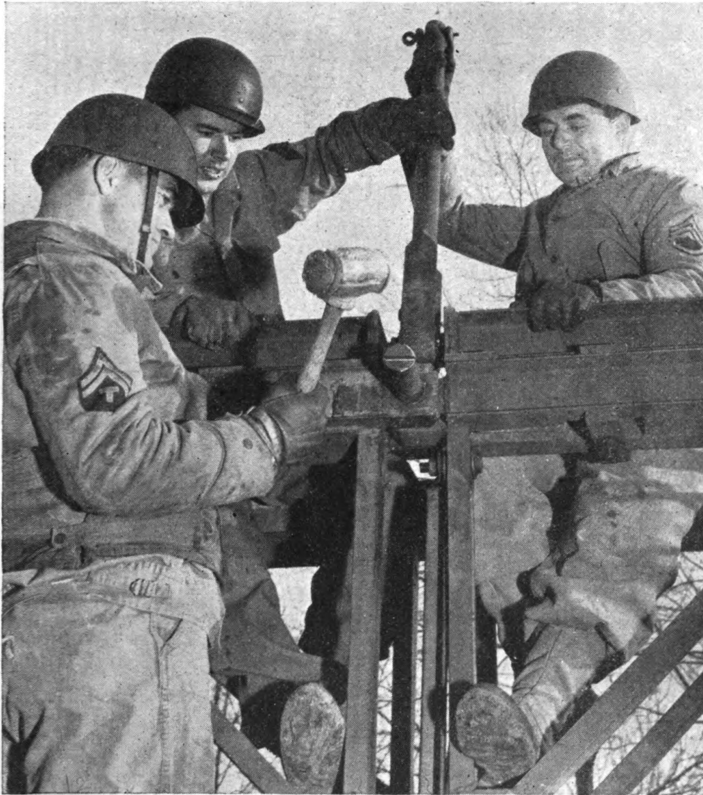
Figure 65.13.—Driving panel pin in second-story panel using chord jack to spread panels.
