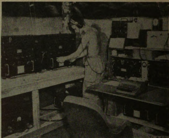
Figure 6-78. H-f radio station consisting of transmitting and receiving components of Radio Set SCR-188.
