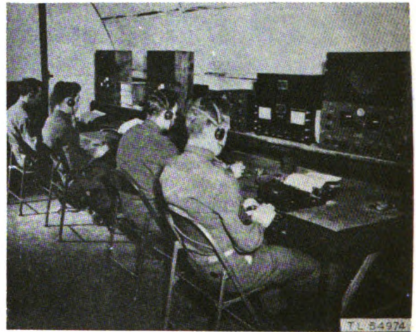
Figure 11-25. Manual Morse code radio telegraph installation.
