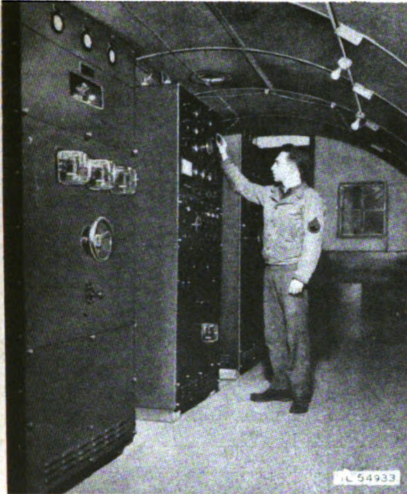
Figure 6-113. Army Communications Service 10-kw transmitting equipment (showing Power Amplifier BC-340 and Radio Transmitter BC-339).
