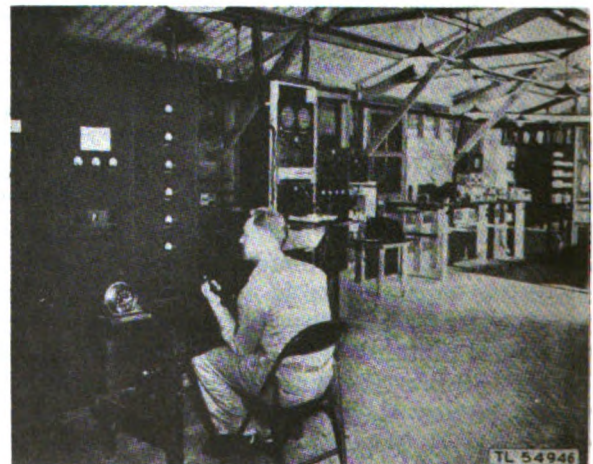
Figure 11-63. Fixed plant radio receiving station, (showing single side band receiver Western Electric Company D-99945 in left foreground).
