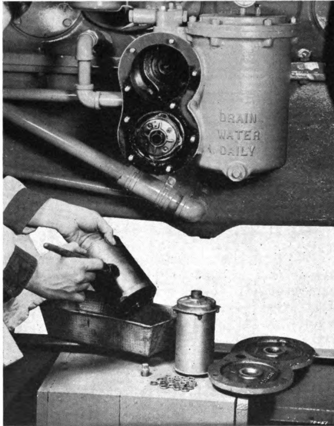
FIG. 24—Cleaning Lubricating Oil Filters
